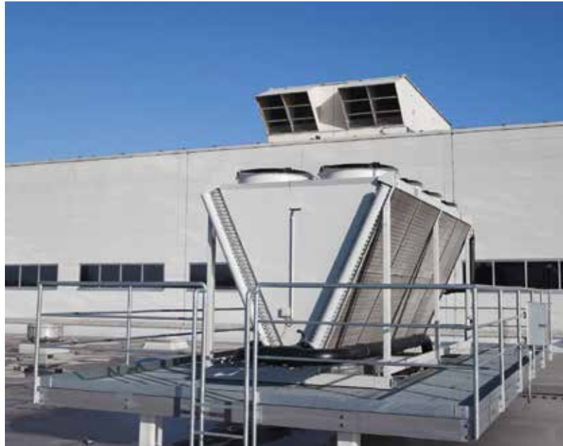
The plastic injection machines at the plant in Neustadt an der Donau in Germany can be completely cooled by means of the free cooler on the roof.
